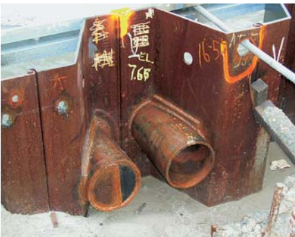
A hole was cut into the piles to pass the rebar tie rods
