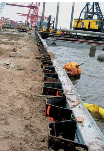
A waling system evenly distributes anchor forces into the sheet pile wall
