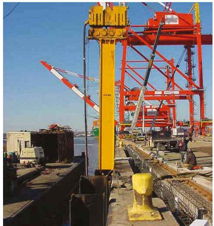
Fig. 12. Installation of AZ below water level with a follower on a vibratory hammer.
