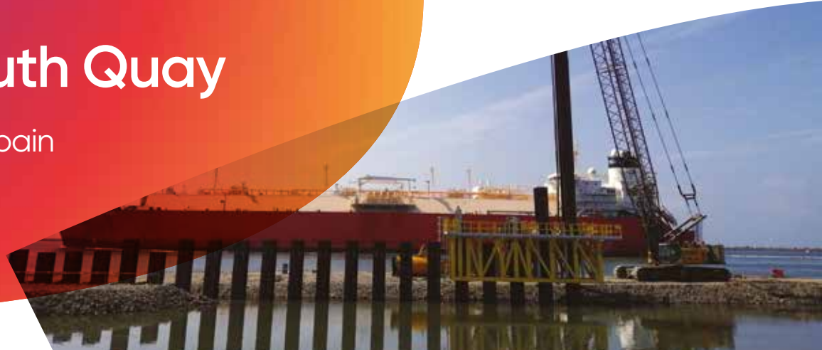
Extension of the South Quay | Installation of the combined wall system HZ ® -M/AZ ® .
