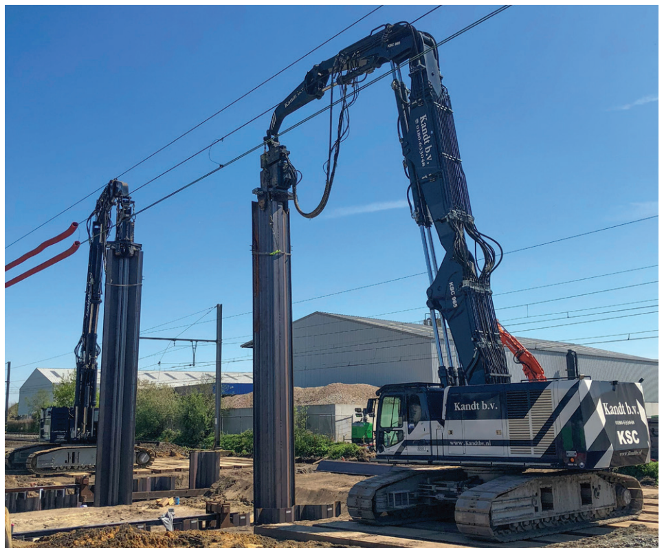
Installation by vibratory hammers with double clamping systems mounted on hydraulic rigs
