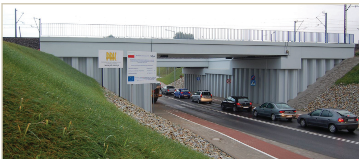
Picture 1. Bridge abutments where traffic loads from the bridge are transmitted to the steel sheet piles.
