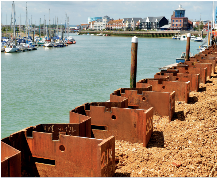
Combined steel sheet pile wall | Tidal Flood Defences River Arun Littlehampton - UK (© High Camera Ltd | UK)
