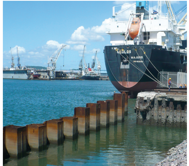
HZ-M / AZ combined wall | Maydon Wharf, Rehabilitation of Berth 12, Port of Durban - South Africa (© Stefanutti Stocks Marine)
