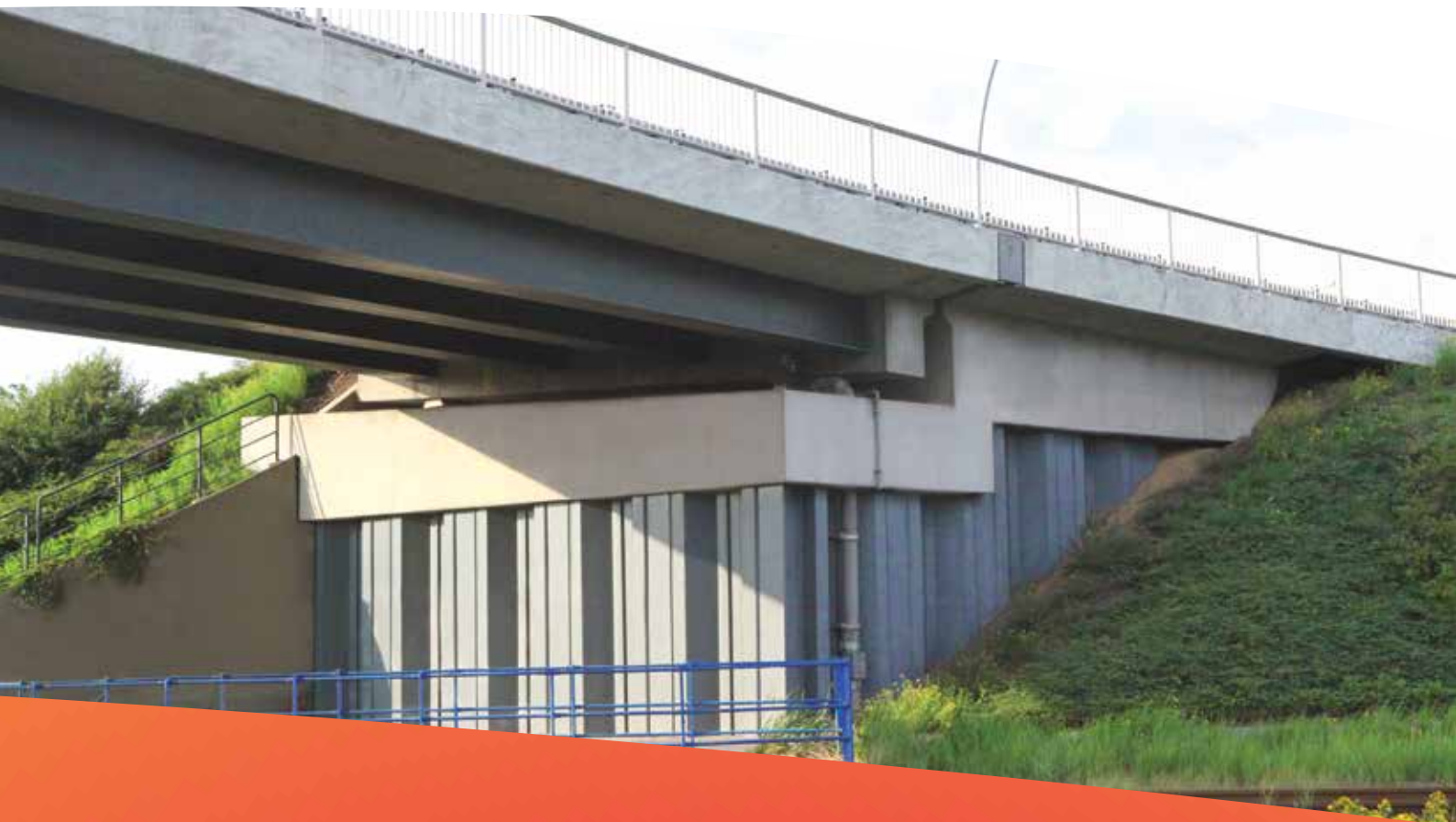
Fig. 3. Example of a conventional road overbridge abutment using combined sheet pile wall (high stiffness) and discrete bearings (Hamburg, Germany).
