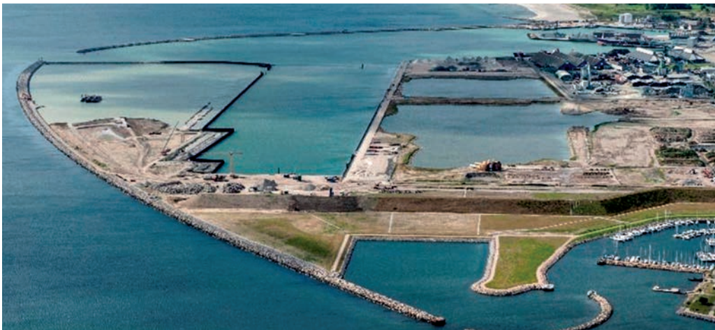
Uniterminal | Port of Koege | Denmark (2016). 4 000 t of AMLoCor © steel sheet piles installed.
