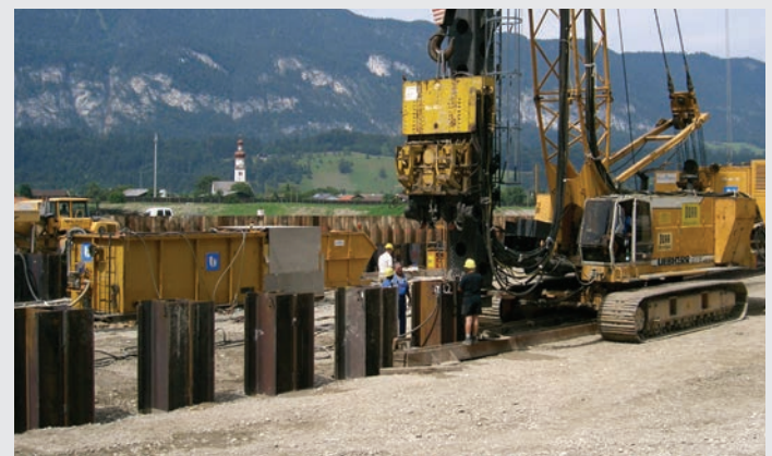
Fig. 18. Template with a single level and piling equipment guided on a fixed leader.
