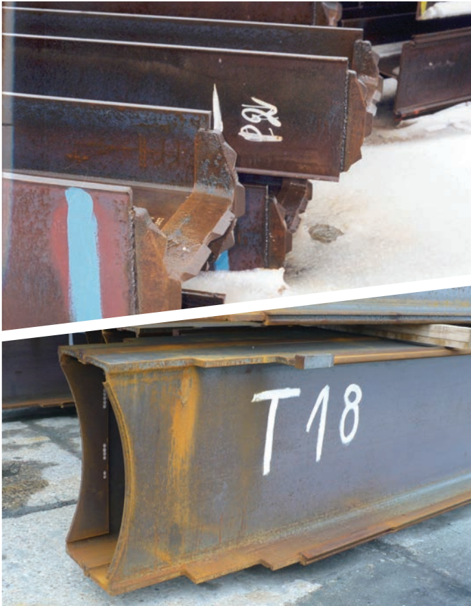
Fig. 24. Reinforcing of the tip of the pile with steel plates / shoes welded on the king pile toe.
