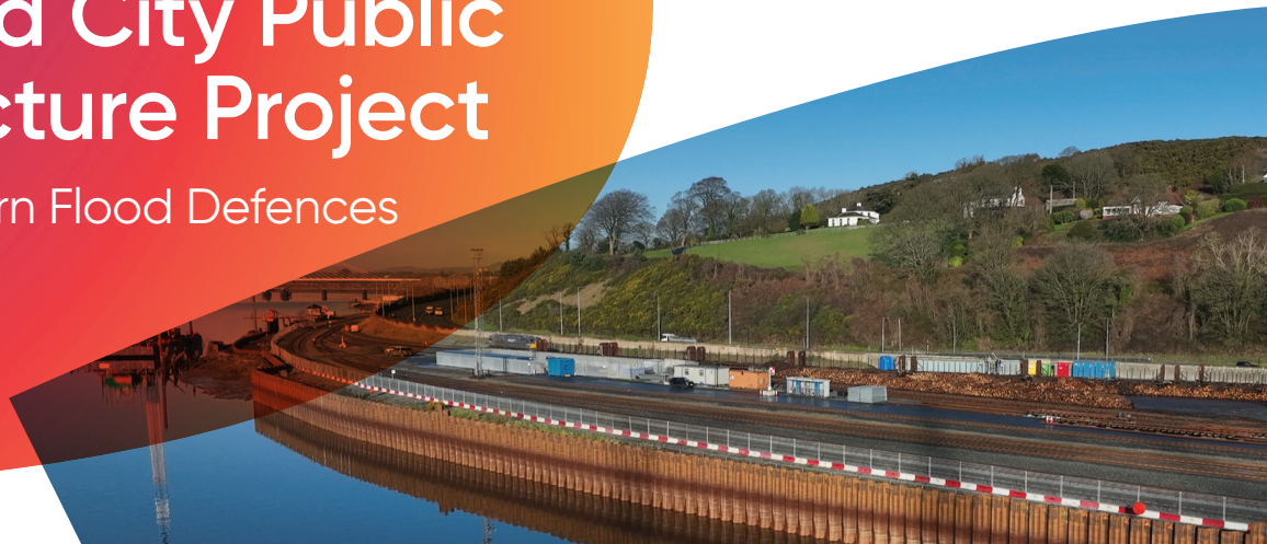
Waterford North Quays Development (Eastern & Western Flood Defences). Retrieved from https://waterfordnorthquays.ie . © BAM Civil Ltd
