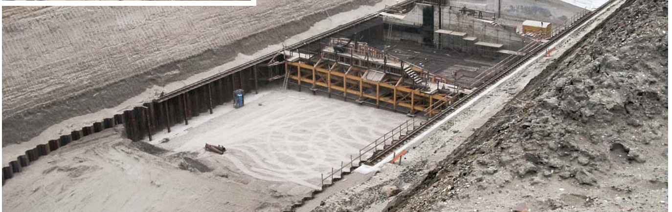
Over 6,000 t of steel sheet piles were used for the foundation of the quay walls
